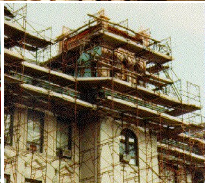
Roof & Cornice Restoration, City of Jersey's City Hall Building – Jersey City, NJ
